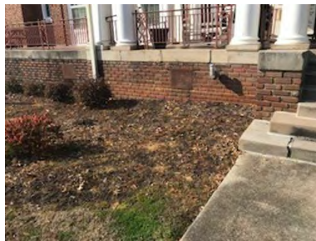
Deteriorating Landscaping, Bare - Joynes
