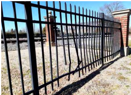
Broken Fence - Alumni Drive
