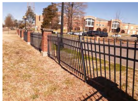
Broken Fence - Alumni Drive
