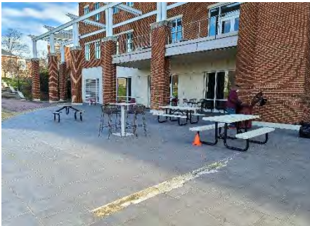
Needed Condition Repair
