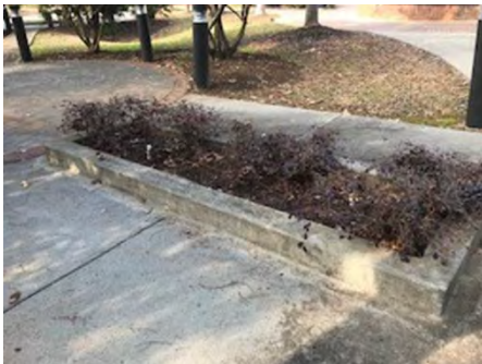
Deteriorating Planting Bed - Hardin Garden
