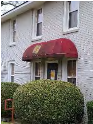
Dirty, Outdated Awning - Shack
