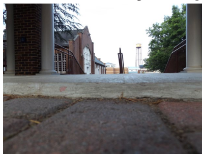
ODS and Facilities Management are constantly monitoring and repairing spots like this one-inch drop on the walkway between Tillman and Margaret Nance. Even something seemingly small can trip up a person using a cane or walker.
