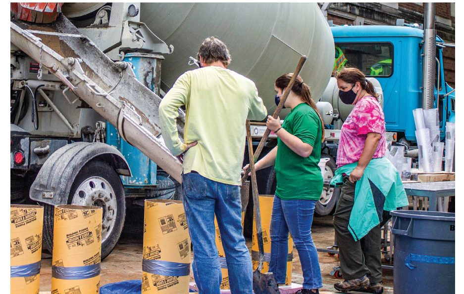
Emily Pilarczyk, middle, oversaw the concrete pouring at the diversity and inclusion garden that she undertook for her Eagle Scout project that is located near Rutledge Building.
